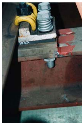
Fig 10: Picture of the resilient rail fastening system after modification of the auxiliary railway bridge [Photo: W. Weißenberger, Müller-BBM]
