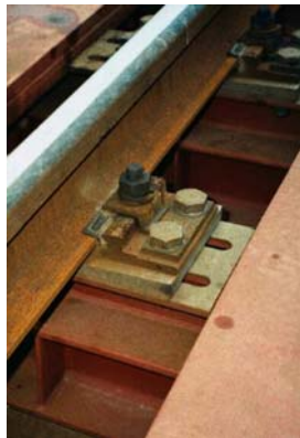
Fig 8: Picture of the stiff rail fastening system in use before modification of the auxiliary railway bridge [Photo: W. Weißenberger, Müller-BBM]
