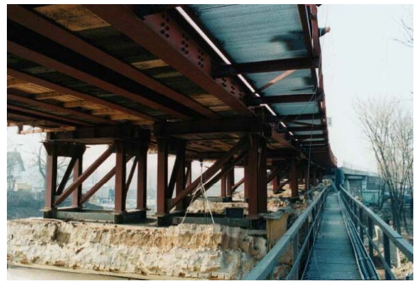
Fig. 6: Underside of the auxiliary steel railway bridge, which has been built on top of the viaduct segments [Photo: W. Weißenberger, Müller-BBM]
